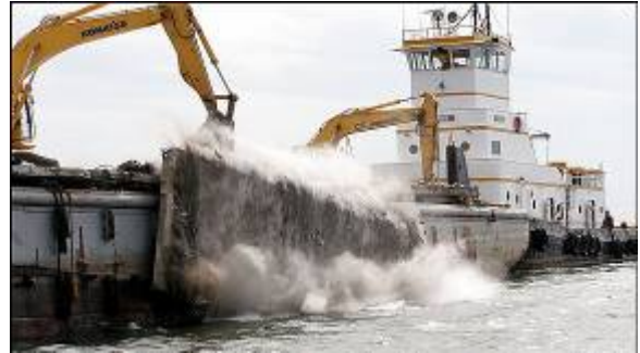
Caption: Rubble from the old Wilson Bridge (I-495) span is placed as artificial reef in the Chesapeake Bay.
